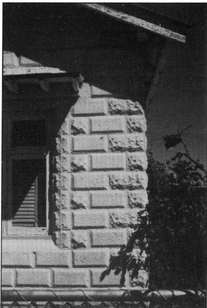
Fig.2 House at Lithgow, NSW. Detail: Cement blocks set as quoins and decorative treatment. (Rusticated pattern.)
